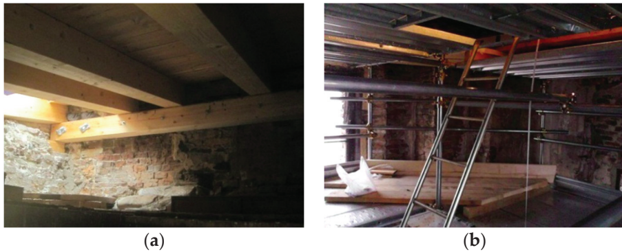
Figure 5. Details of (a) the added wooden roof and (b) the provisional scaffoldings.
